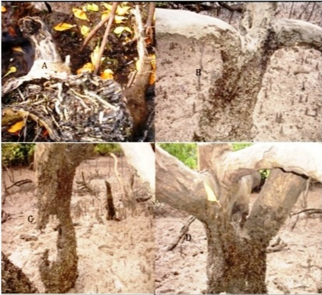
Figure 3. Mangrove wood deterioration by borers. A: Heavily fragmented piece of wood with vacant tunnels created by extensive terenid boring activity. B, C and D, tree trunks severely damaged by isopod borers.
